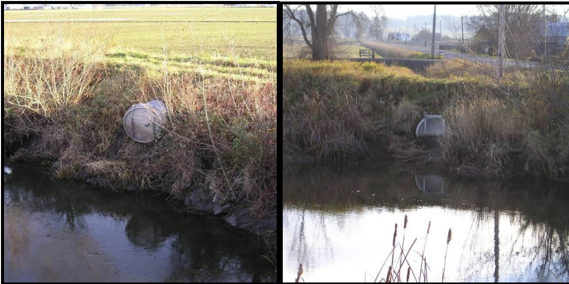
Figures 1-2 & 1-3 Floodgates, Drainage District 25 – Samish River system.
