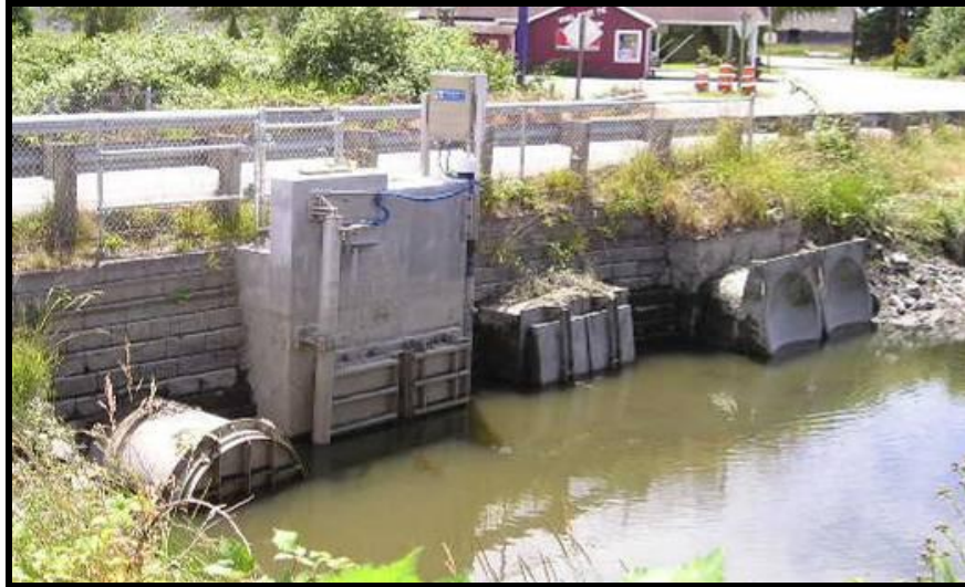
Figure 1-1. Tidegates on Edison Slough, various top-hinged gates and a Self Regulating Tidegate (center left). County maintained tidegate complex.
